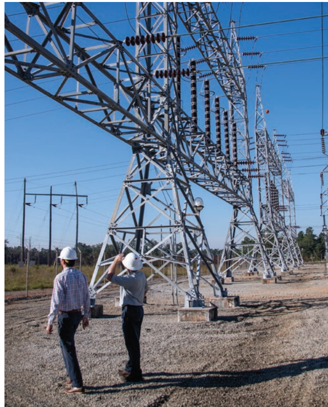
SRNL power substation. (SRNS Photo)
